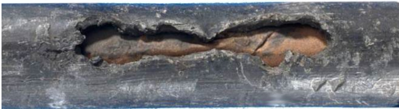
Lead sheath corrosion on a PILC cable
