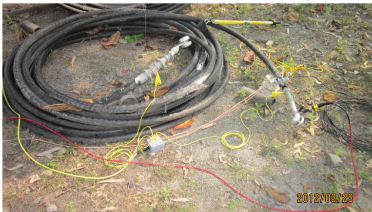
Figure 64, connection arrangement with guard ring and corona hoods, VSE box, Frida TD connection
