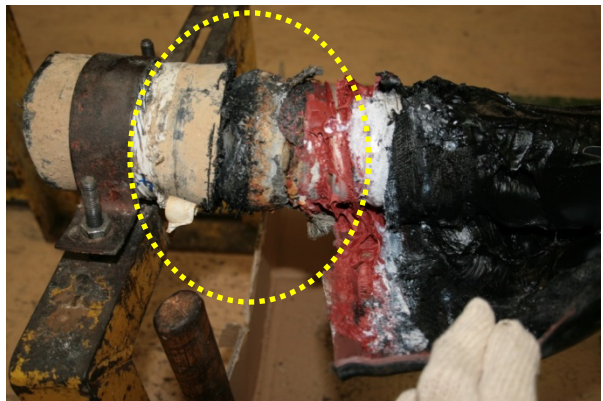
Water found in cable during joint recovery. CAS corroded at Sumitomo cable side inside inner sleeve
