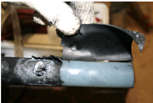
Water sign noted in insulation screen
