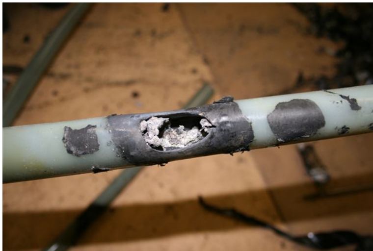
Cable body fault, L2 at 125m
