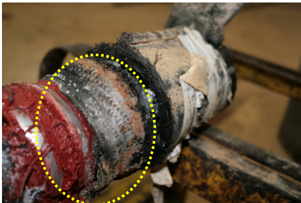
Fault point on L3 at Sumitomo
