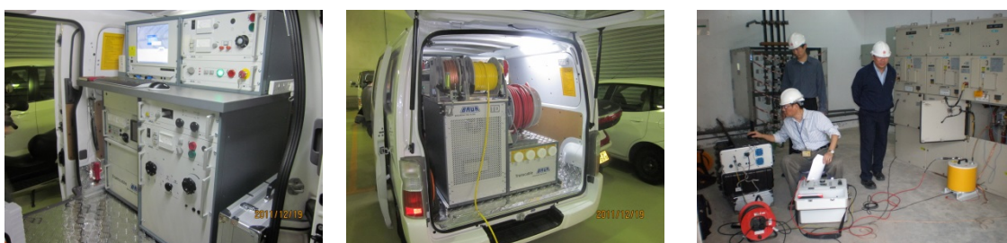
Figure 108: BAUR VLF TD / PD Systems used
