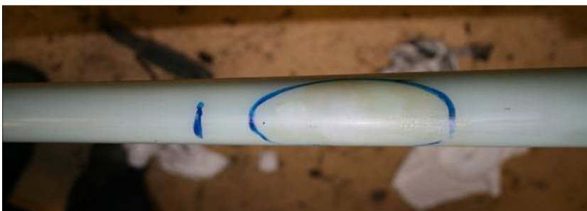
Visible white spots after removal of semi conductive layer, section #1
