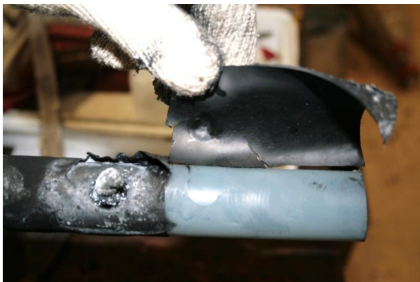
Water sign noted in insulation screen
