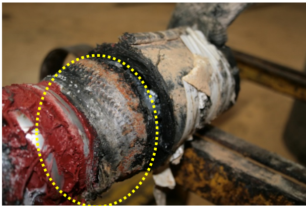
Fault point on L3 at Sumitomo
