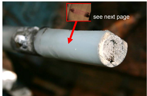
Suspected water tree developed near to fault point
