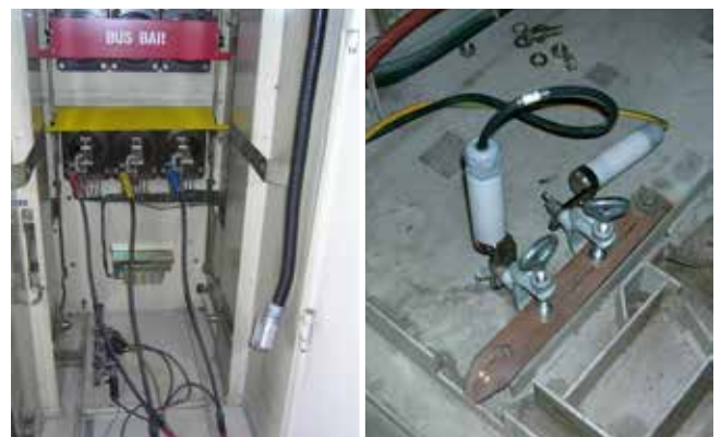
➤ 3 phased connection, common grounding point of safety earth and operation earth clamps
