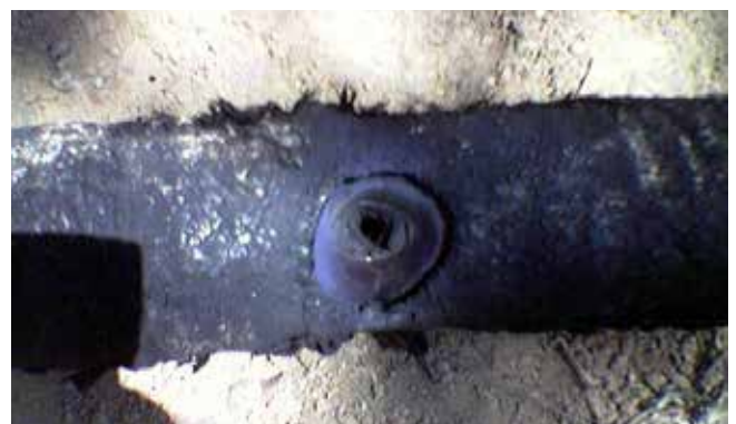
➤ Cable Fault in a 132 kV PILC cable
