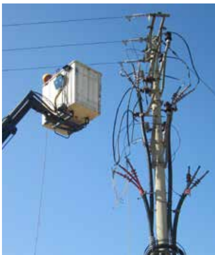
➤ connection to pole mounted cable terminations
